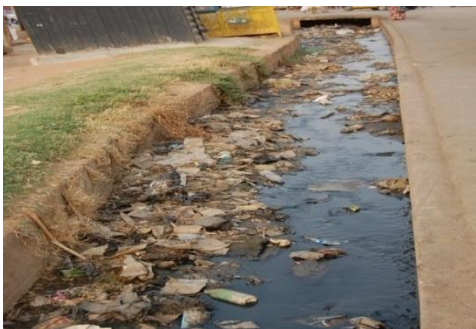
Plate 1.4: Blocked Drainage in Zone M.
