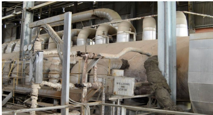
Figure 2: Boiler Drum (Ajaokuta Steel Power Plant)
